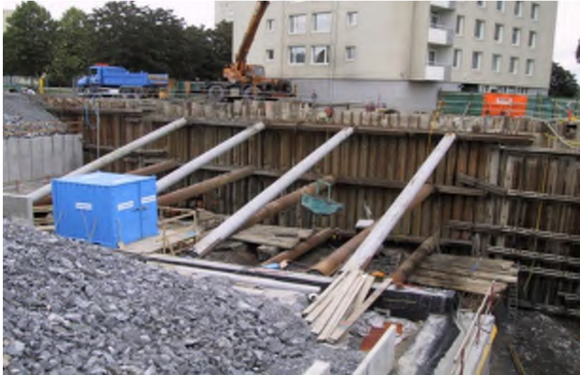
Figure 19: The sheet pile wall close to the residential block “Asplången” (Carlsson et al. 2004).
